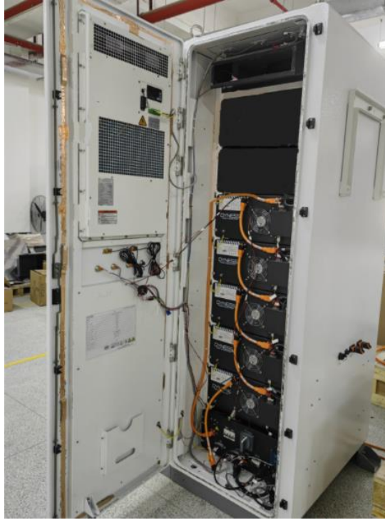
铭牌, 电池柜 (label, Battery cabinet) -6
